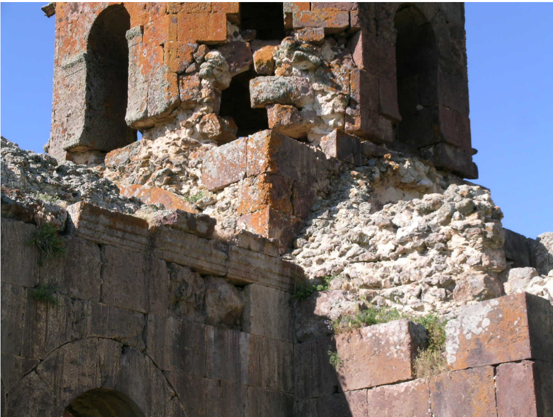
Fig. 6. Same, detail of exterior from the southwest at the corner of the nave and transept (author)
